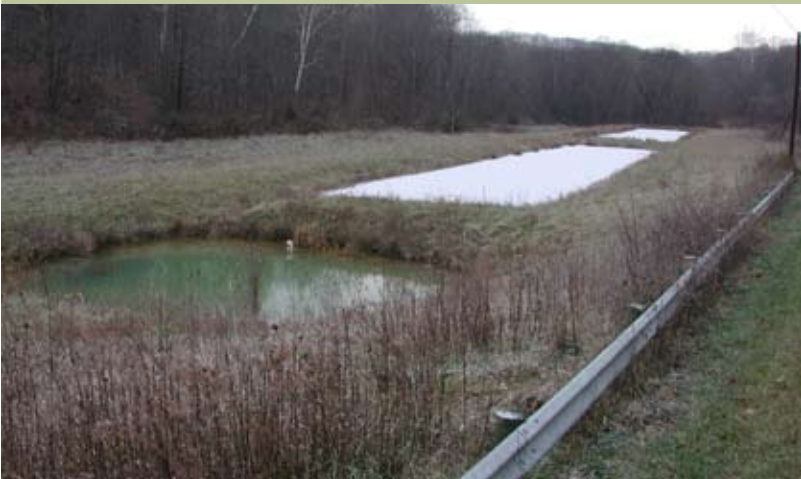
Successive Alkaline Producing System (SAPS) Photo by Ben McCament
